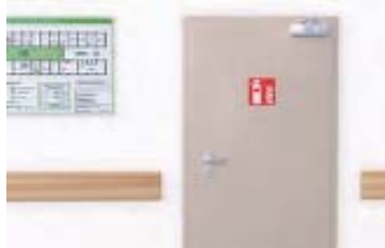
Fire protection doors
